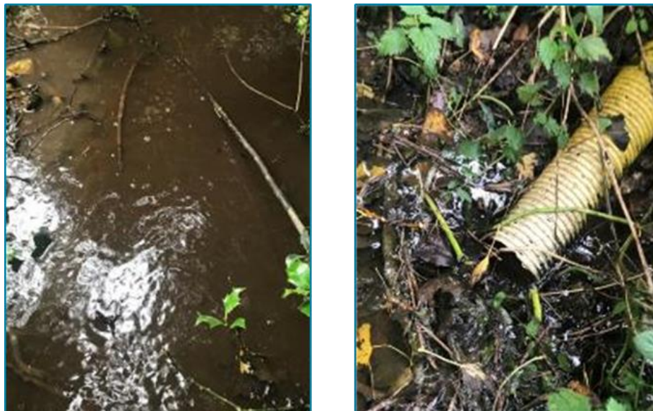
Plate 20.3.8: Silt deposition and outfall pipe.
